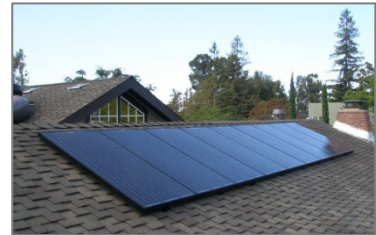
Figure 3.2 Building-mounted solar energy system
